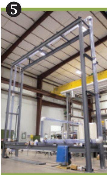
5 Fabricating and commissioning the Pipe Flow Loop for two-phase flow regimes in thermosiphon piping
