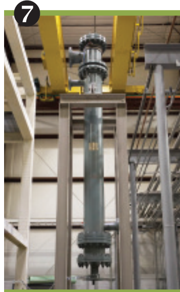
7 Installing and shakedown testing of the new thermosiphon reboiler in the Prototype Test Unit
