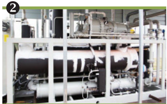
2 Purchasing and installing a 60-ton chiller, which will expand the test temperature ranges of our current rigs
