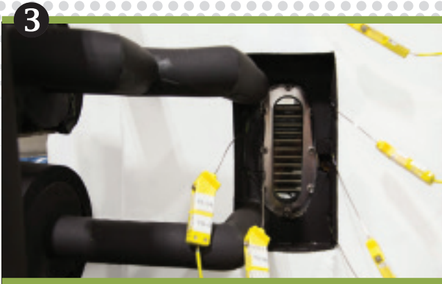
3 Installing and commissioning the shellside test section for the Low Pressure Condensation Unit, which has a window for visualization studies
