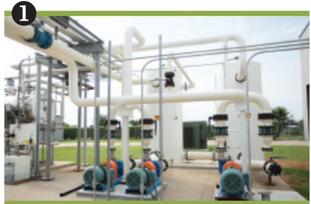
1 Commissioning the Liquid-Liquid Heat Exchanger test rig, followed by 14 audit and certification tests for The Air-Conditioning, Heating, and Refrigeration Institute (AHRI) certification program
