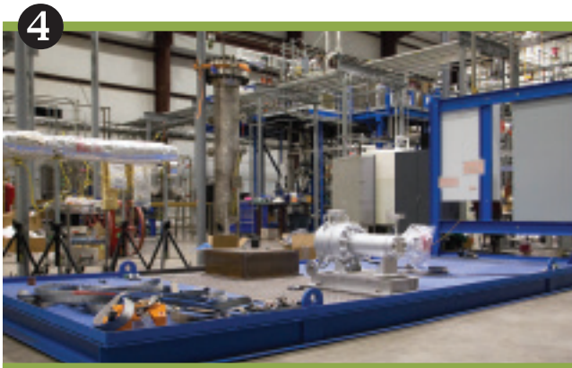
4 Constructing and commissioning the second High Temperature Fouling Unit to increase the capacity of our crude oil fouling test program
